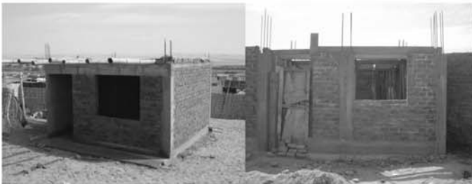
Two homes that are nearing completion in Pisco, Peru for Earthquake victims.
