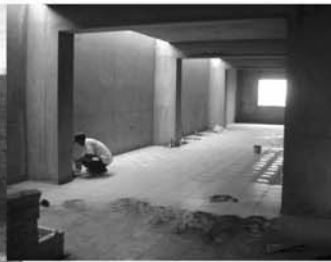
Tile being put down in the Bible School & Mission Training Center in Lima.
